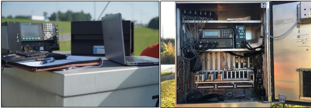
Figure 23: Traffic Signal Controllers
